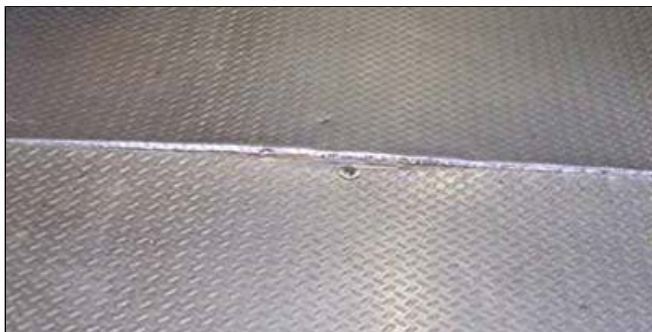
Heavy cart traffic or shelving can result in floor delamination.
