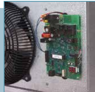
One Master Controller board (shown with cover off) is mounted to the evaporator coil in the ante-room.
