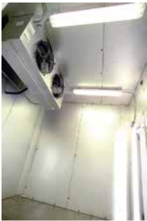
Plasma and storage freezers maintain a consistent -40°F.
